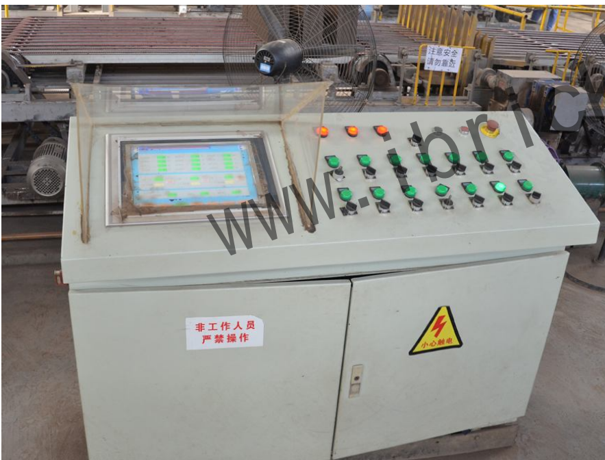
Operating floor for brick separating and transporting control system
