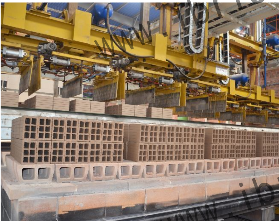
Working condition of full-automatic brick stacking machine
