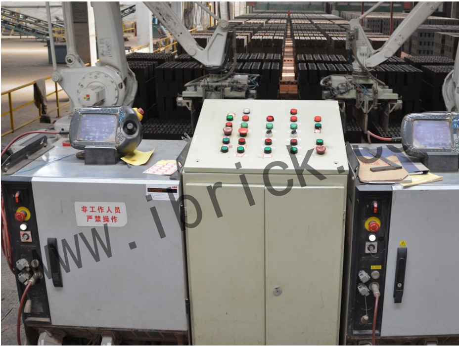
Control system of robot stacker
